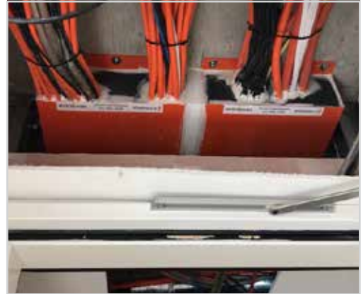
Double Vertical FyreBOX installed above a doorway to allow for the provision of large amounts of services in a small space.
