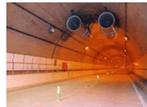
Electrostatic Precipitator - Tunnel Ventilation
