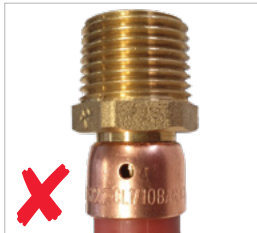
Witness hole not completely filled
