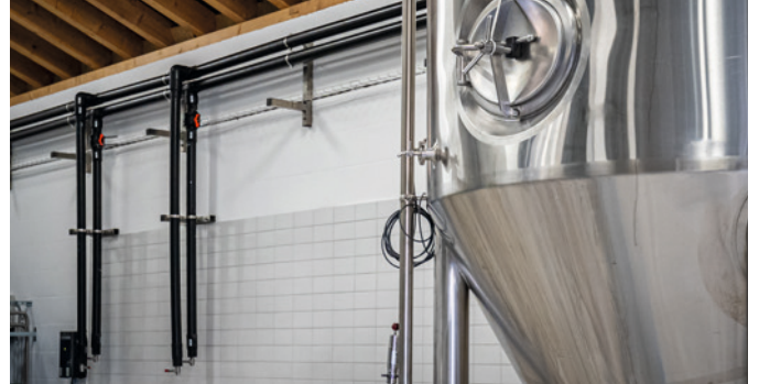
The two master brewers were able to cut the already pre-insulated plastic pipes and install them in a single session as desired without any previous expertise.
