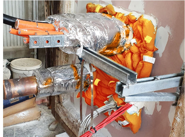
Image: Metal Pipes up to 100mm, unwrapped bundles of small cables and cable trays
