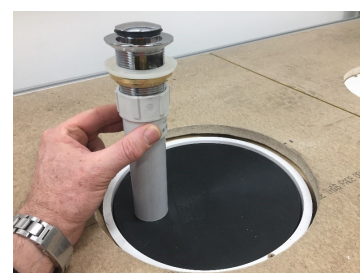
Waste pipe into smart seal
