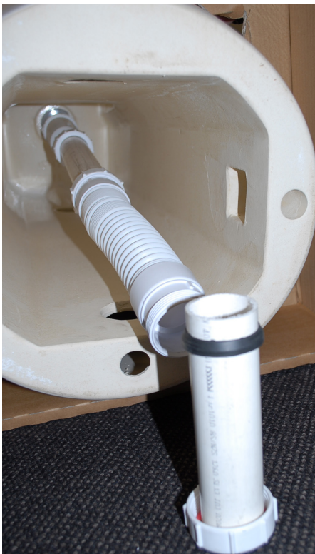
Fig. 3: Access under basin showing connection of flexible waste hose (provided) to 40mm PVC DWV in floor
